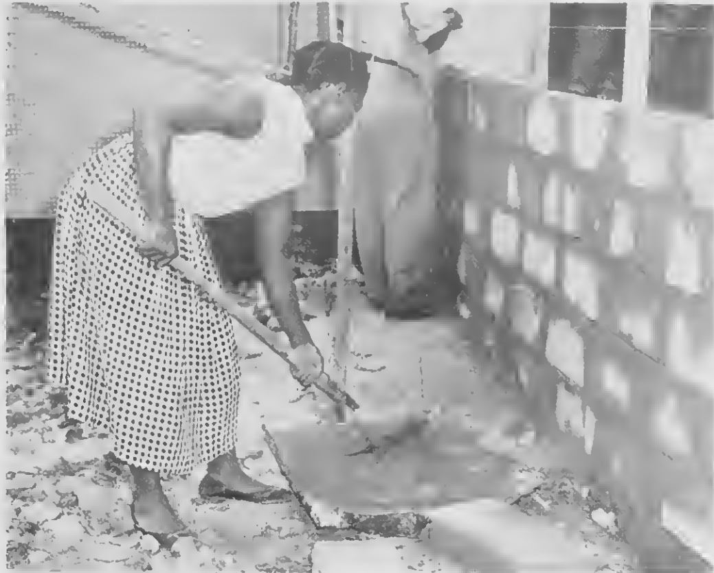
THE ENTIRE building was covered with cement stucco. That much material needed a lot of mixing. The women helped.
